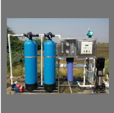
Industrial RO Plant
