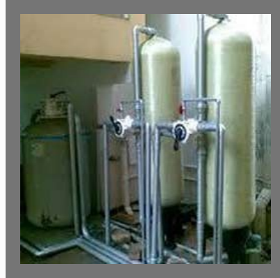
Iron Removal RO Plant
