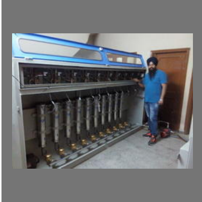
Silver Ionization Plant
