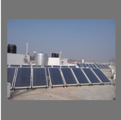
Solar Water Heating System
