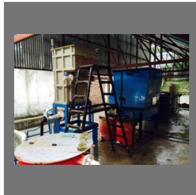
DCI Sewage Treatment Plant
