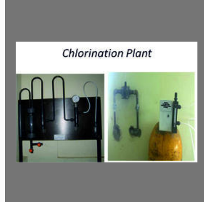
Gas Chlorination Plant
